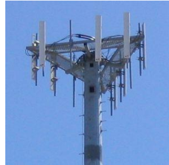
Top of a cellular radio tower
